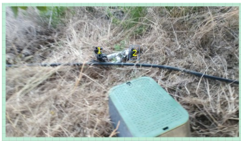
Figure 3: Orchard sprinkler (one zone not used)
