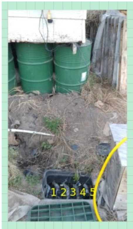
Figure 8: Garden sprinkler valve box
