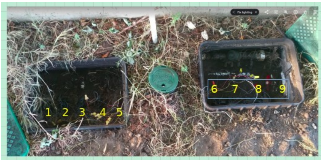
Figure 1: This shows the boxes by the west end of the garage. Numbers are shown in yellow.
