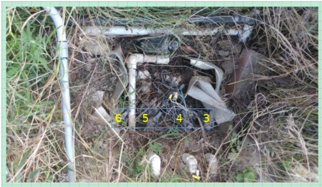
Figure 5: Sprinkler box outside the greenhouse.
